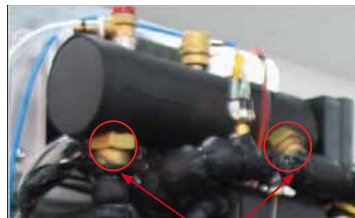
Water piping nuts
